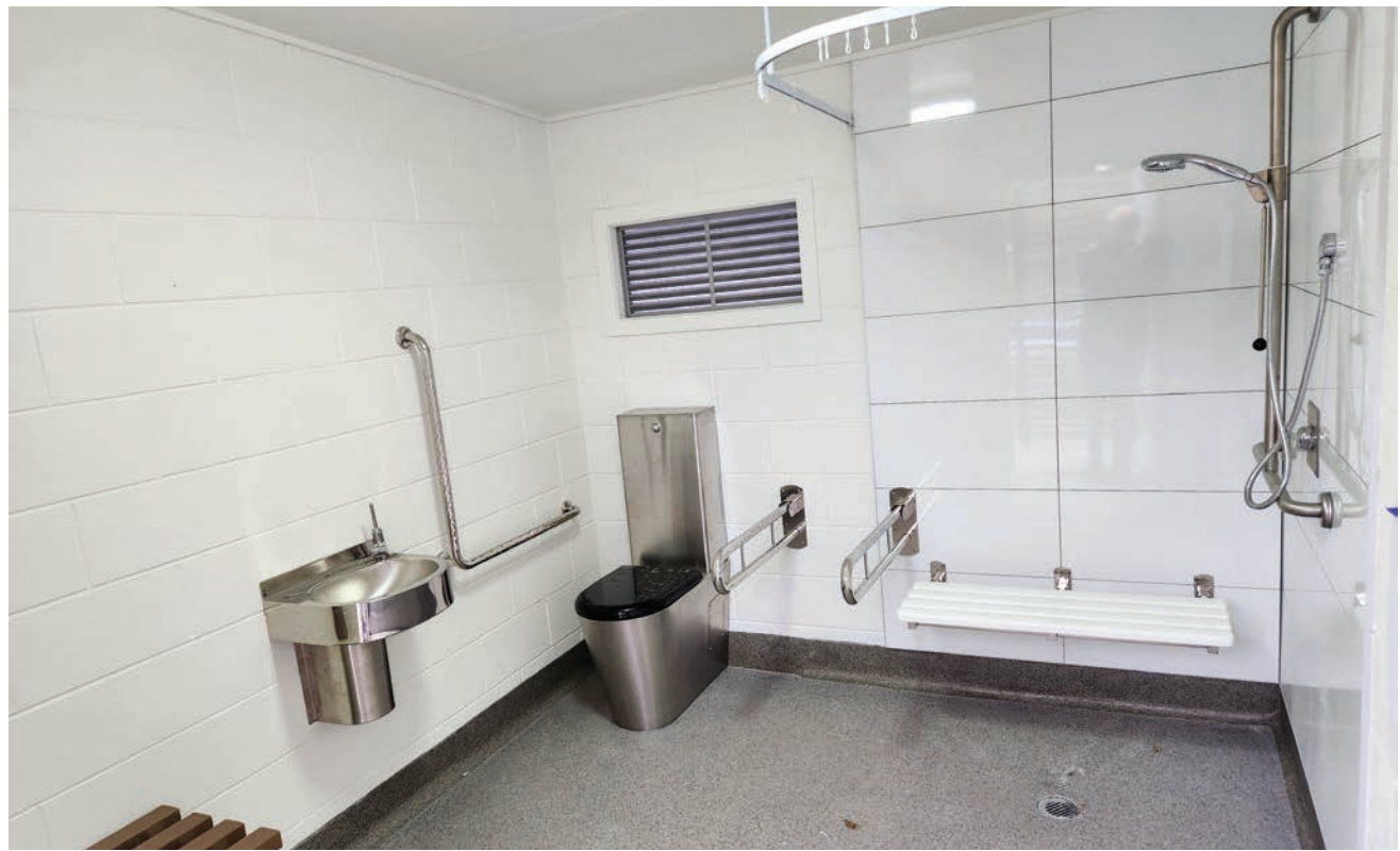
A new toilet block at Okato Pool will make it easier for those with limited mobility.
